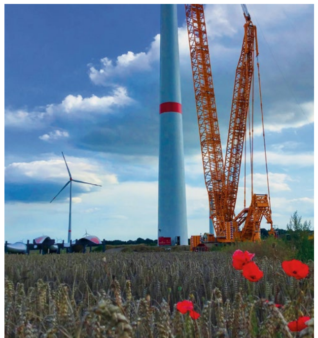
Quelle | Source: eno energy
