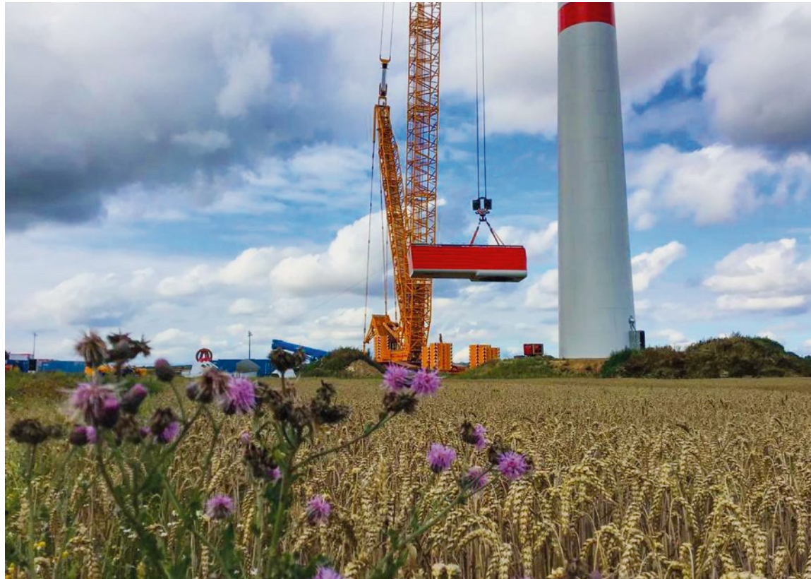
Quelle | Source: eno energy
