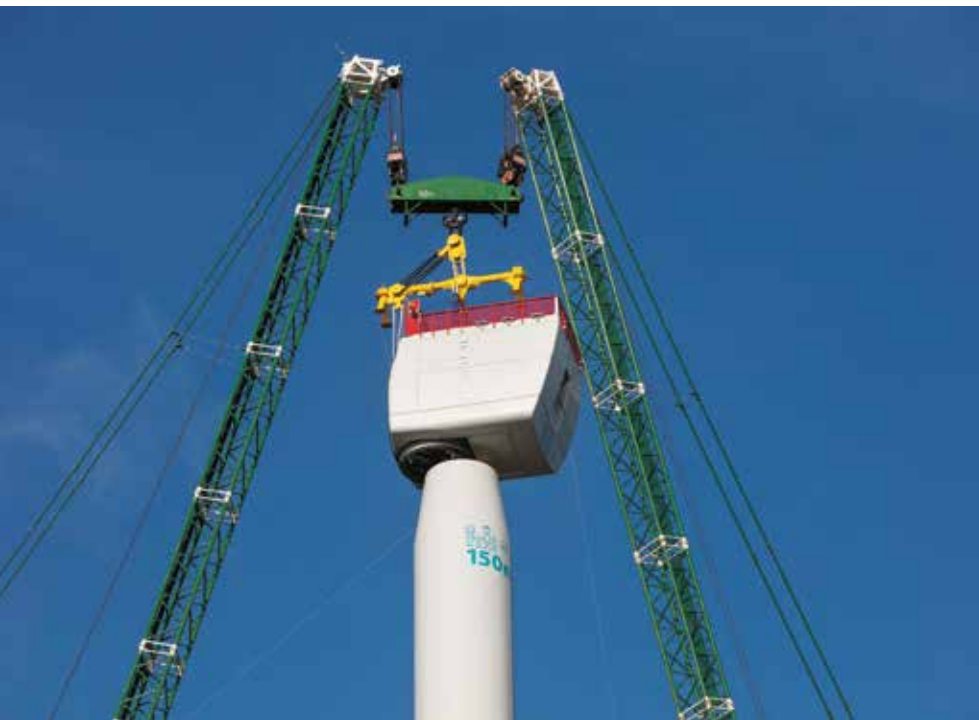
Quelle | Source: Siemens Gamesa Renewable Energy
