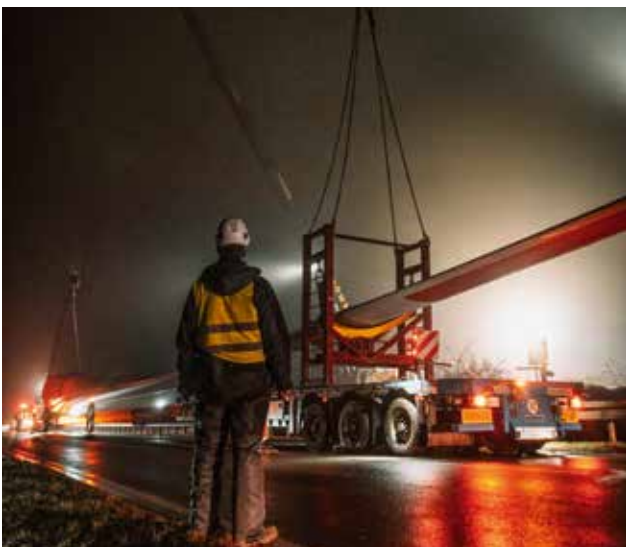
Quelle | Source: eno energy
